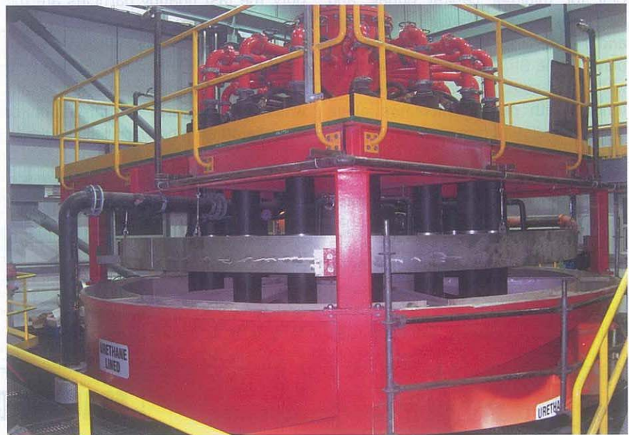
The newly installed B5400/18 Jameson Cell used for Prefloat Concentrate Cleaning at Red Dog Mine, Alaska
