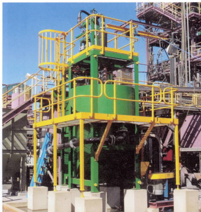
Xstrata Technology's latest IsaMill and Jameson Cell installations operating at the Cosmos Mine in Western Australia.
